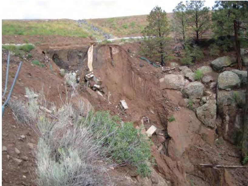
Figure 4.29. Landfill Sedimentation Pond Erosion
