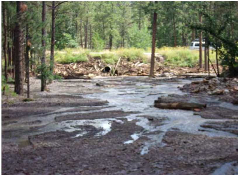
Figure 4.26. Six-Foot Deep Gravel and Mud Covering Drainage Inlet at Ponderosa Estates.
