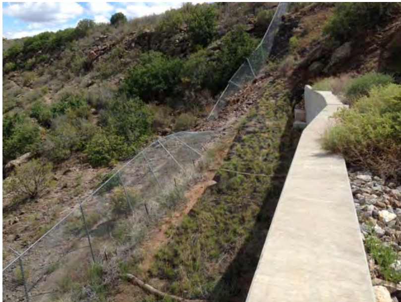
Figure 4.32. Debris/Fence Damage at Airport
