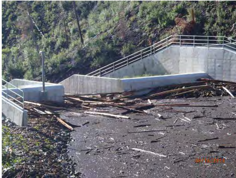
Figure 4.33. Debris at Los Alamos Reservoir Spillway
