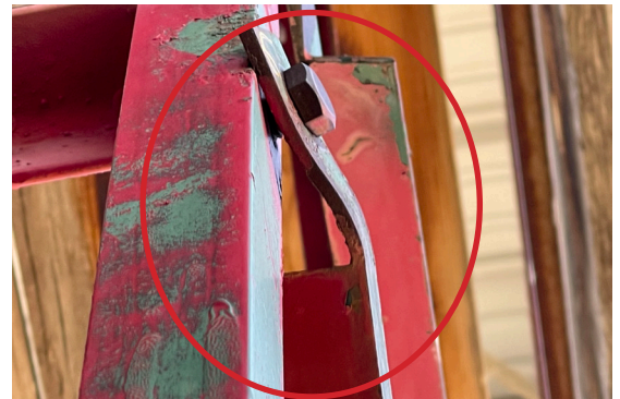
View of failed connection
