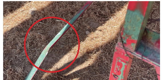
View of structural member buckling failure
