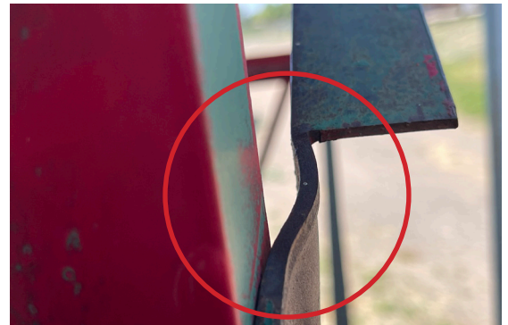
View of buckled connection
