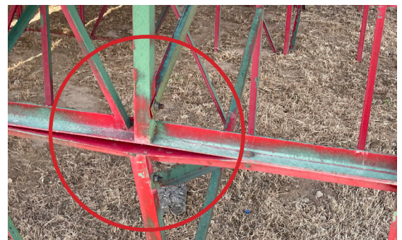
View of prying failure
