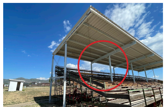
View of missing cross bracing cables
