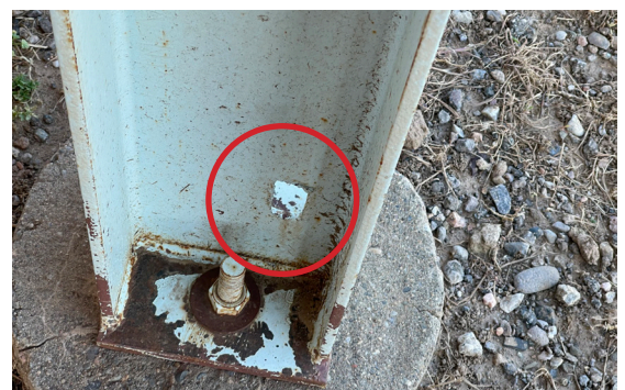
View of missing cross bracing
