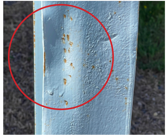
View of column buckling
