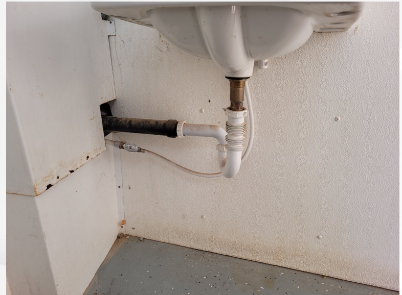
Pipes lack insulation
