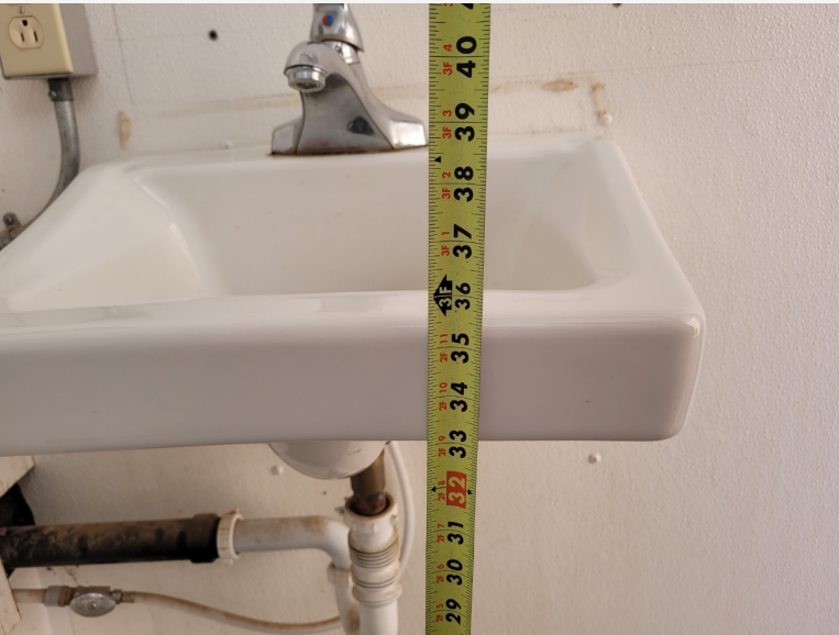
Lavatory mounted too high
