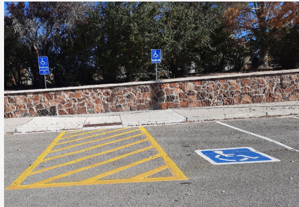
Parking stall/aisle slopes too steep
