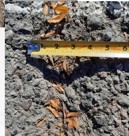
Accessible surface in disrepair
