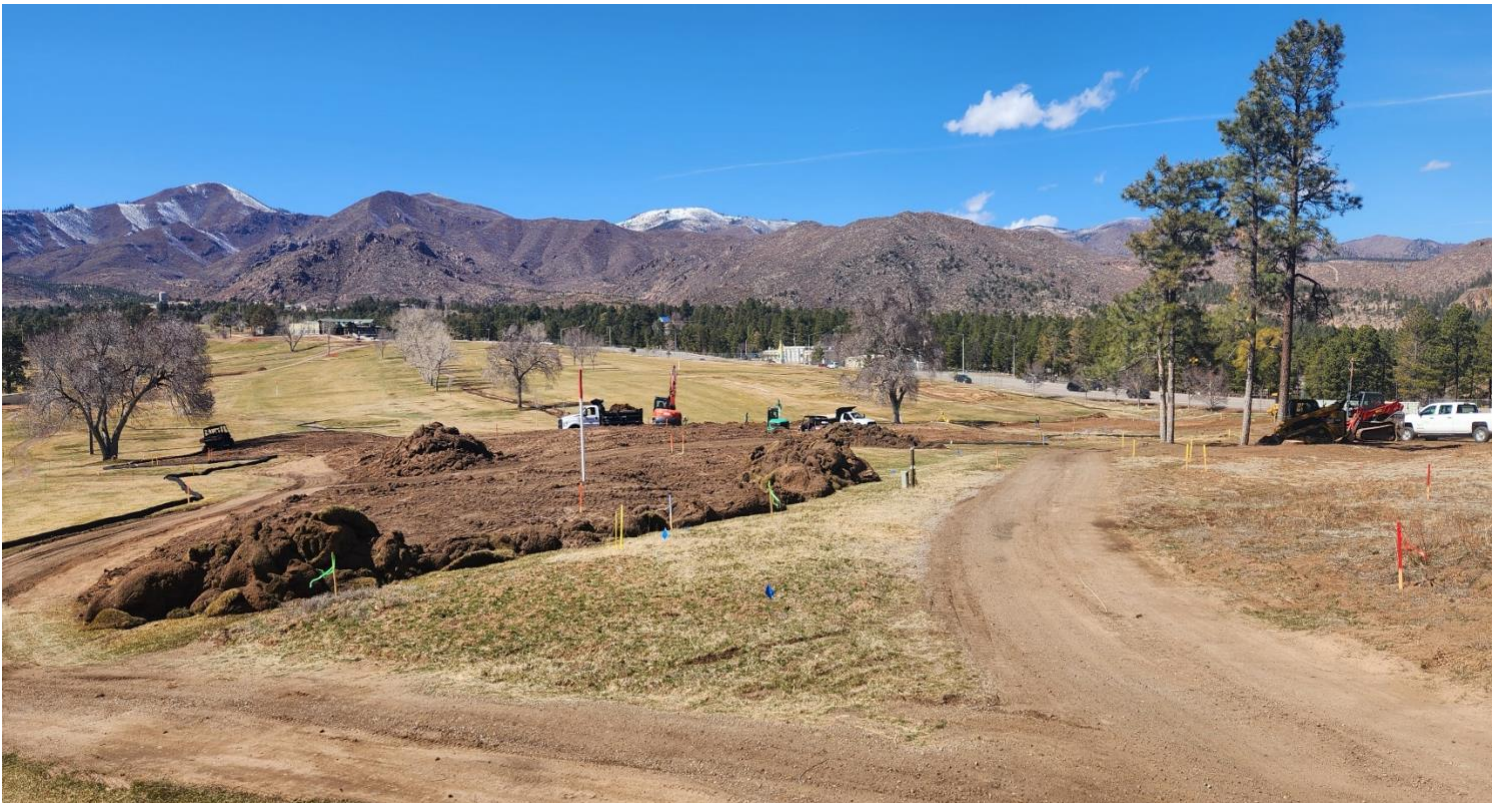
NEW #9 TEE COMPLEX BEING BUILT VIEW FROM BEHIND THE NEW COMPLEX AREA, FACING WEST
