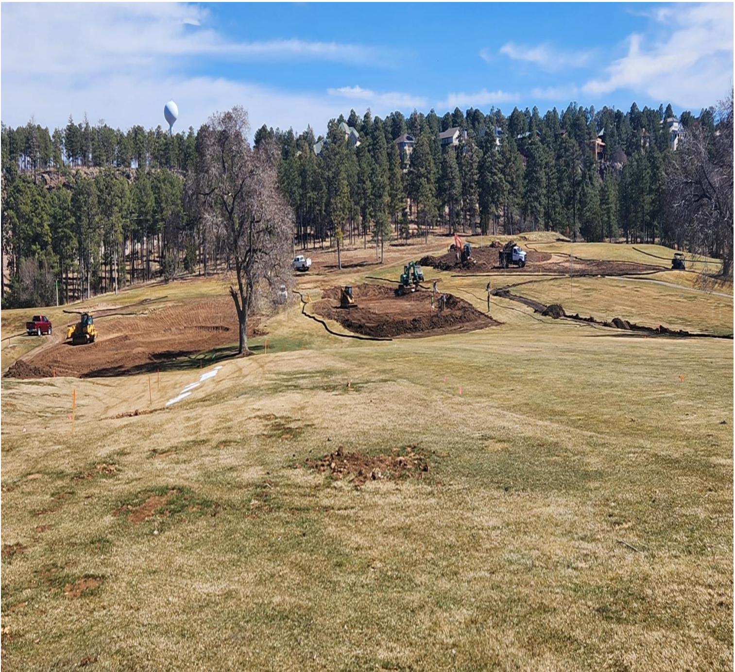
NEW #8 GREEN FAR LEFT IN PHOTO OLD #8 GREEN, CENTER IN PHOTO, THIS AREA WILL BE NEW #7 TEE COMPLEX #9 TEE COMPLEX BEING REBUILT, FAR RIGHT IN PHOTO
