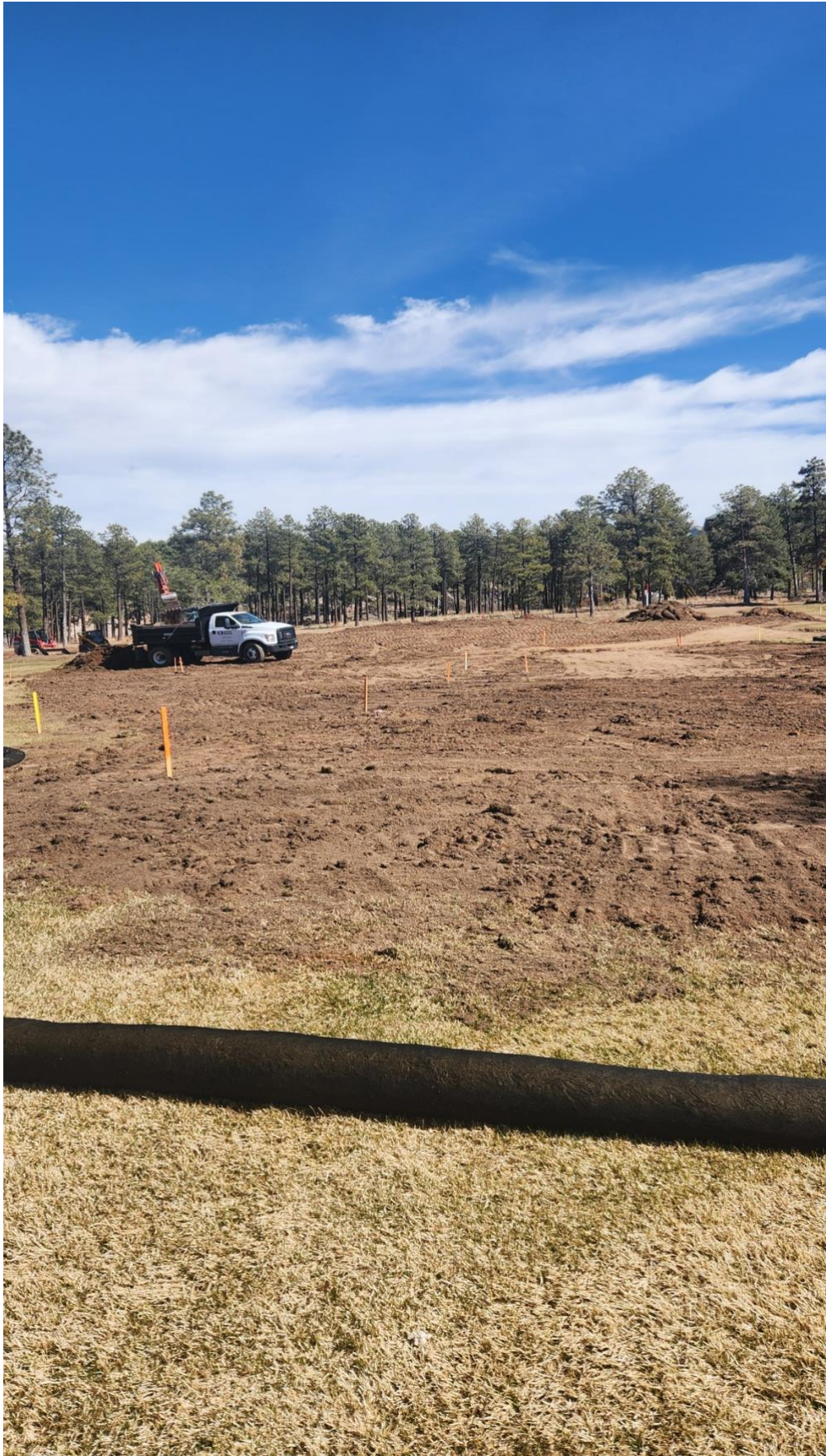
HOLE #9 NEW TEE COMPLEX BEING BUILT VIEW FROM FRONT OF COMPLEX FACING EAST
