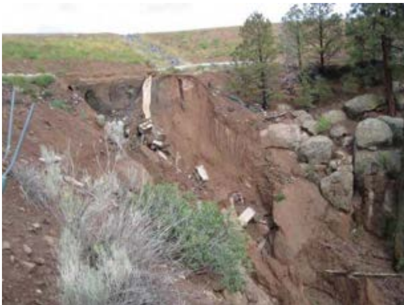
Figure 4.29. Landfill Sedimentation Pond Erosion
