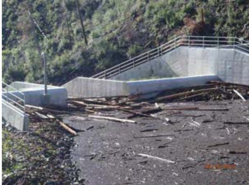
Figure 4.33. Debris at Los Alamos Reservoir Spillway
