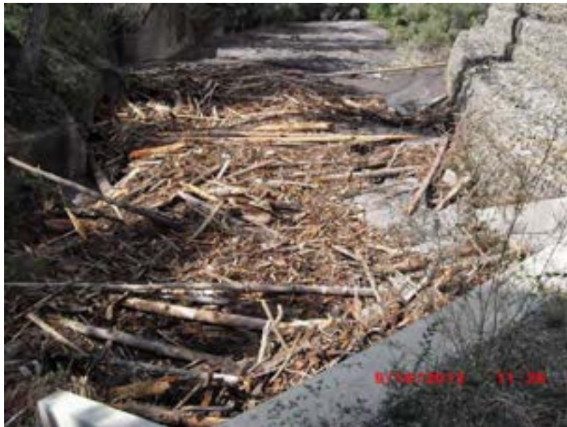
Figure 4.27. Timber, silt and debris blocking box culvert inlet on North Road
