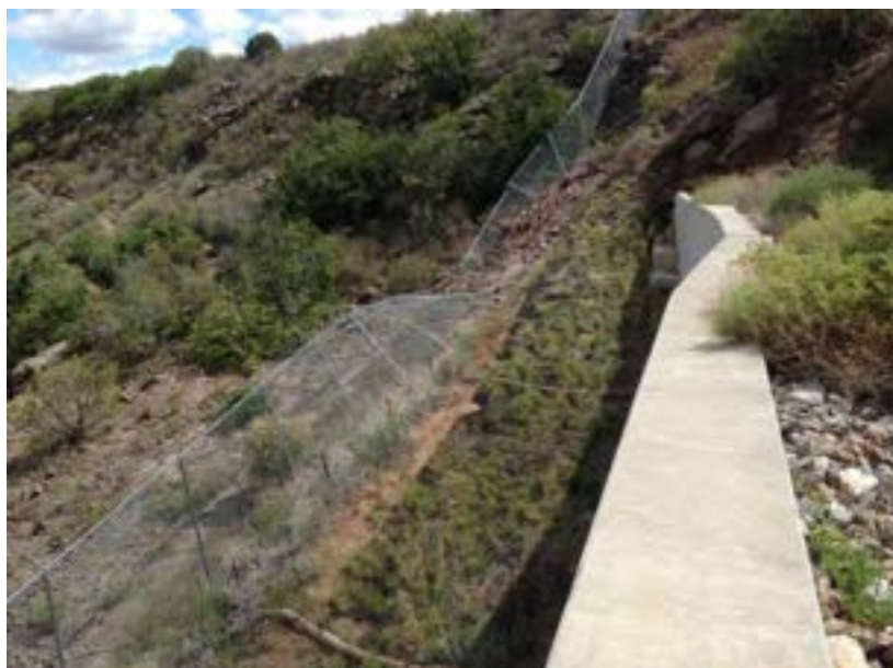
Figure 4.32. Debris/Fence Damage at Airport
