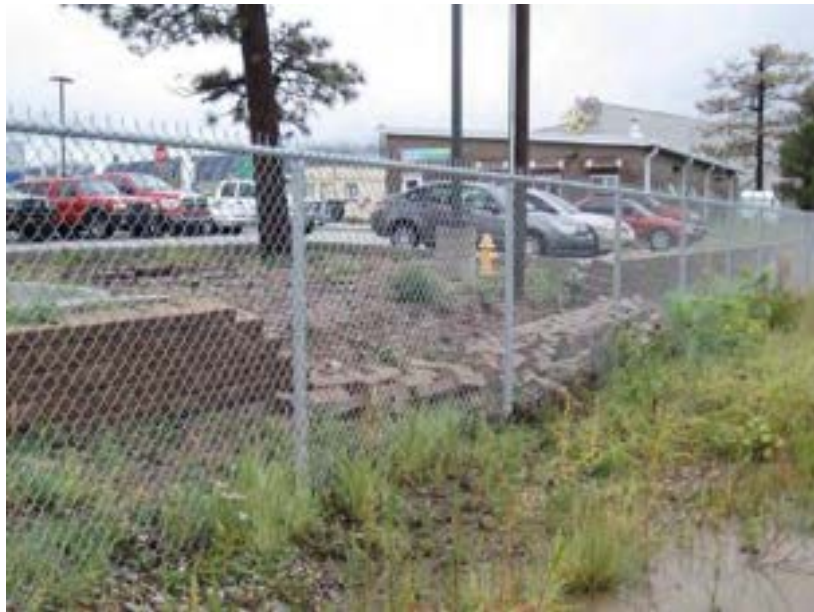
Figure 4.31. Damage to Retaining Wall at ECO Station
