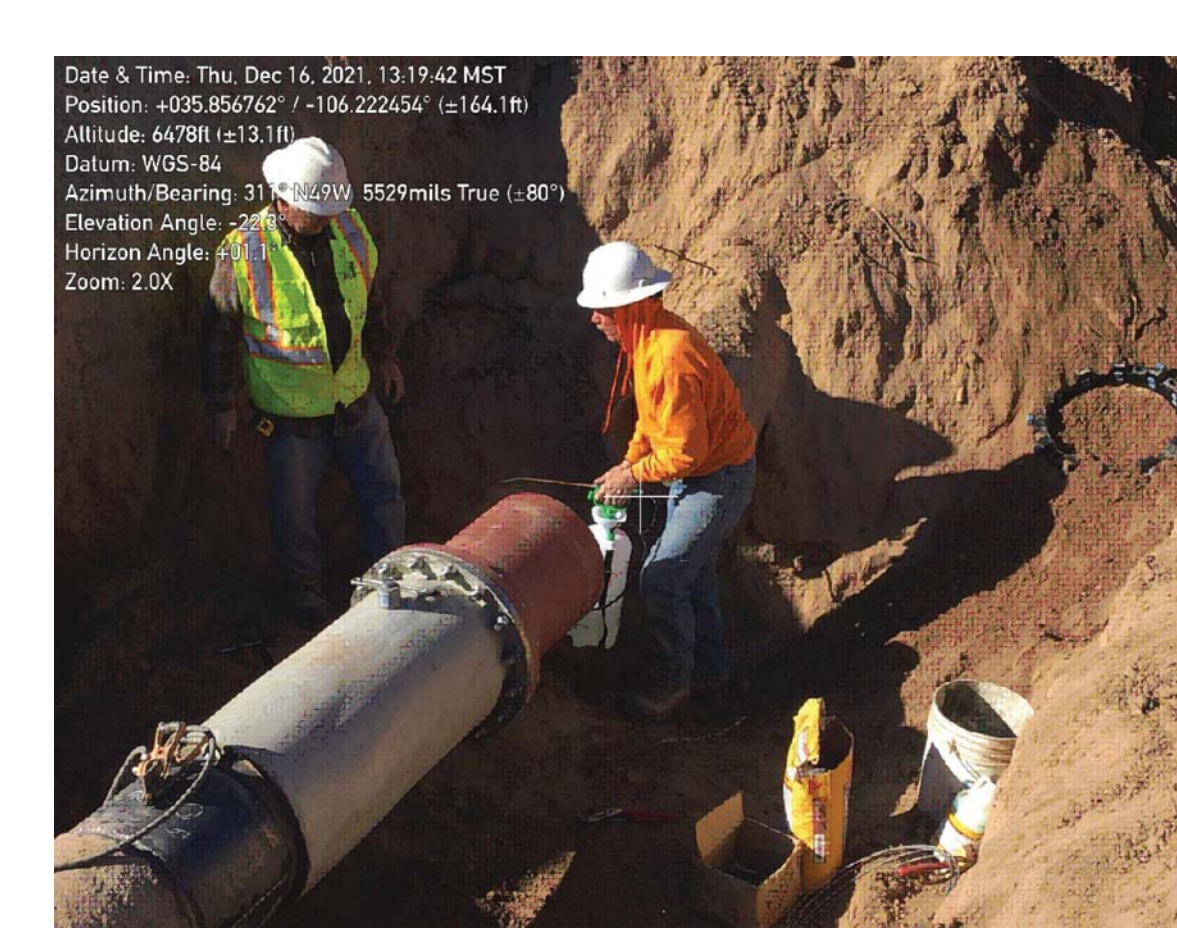
SOUTH NM4 EXISTING CONNECTION DETAIL STA: 0+00 16" CCP TO DIP TRANSITION FITTING TO SALVAGE NOT TO SCALE
