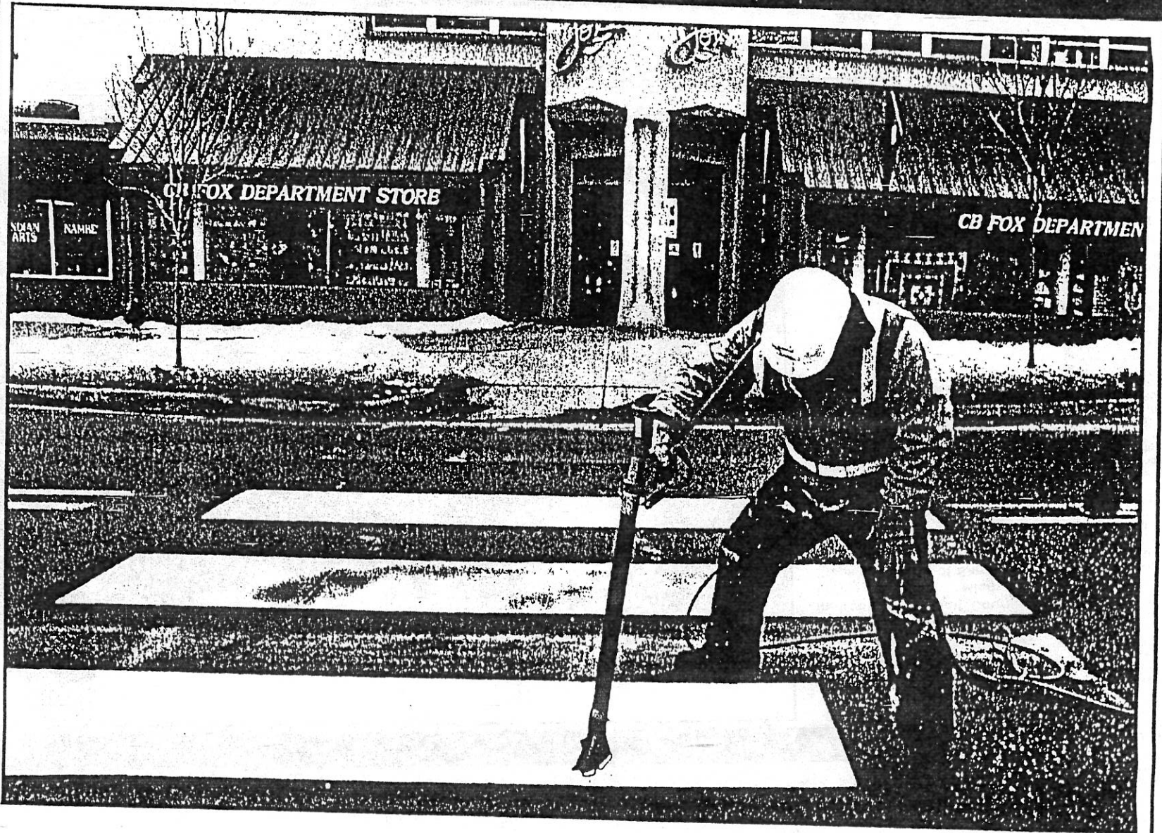
Downtown on Central Avenue, Los Alamos County employee David Rodriguez applies heat to thermo-plastic strips that will
